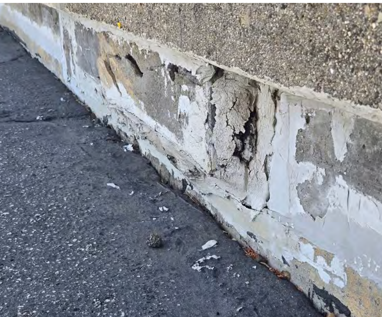
Figure 7: Fractured seismic shear key, east side of North Wall at Equestrian (should be replaced)
