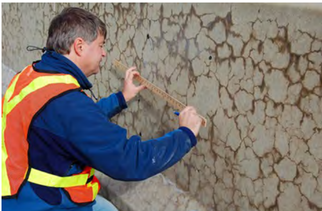
Figure 1: Example of Advanced Alkali-Silica Reaction. This picture is NOT from a LVMWD Facility.
