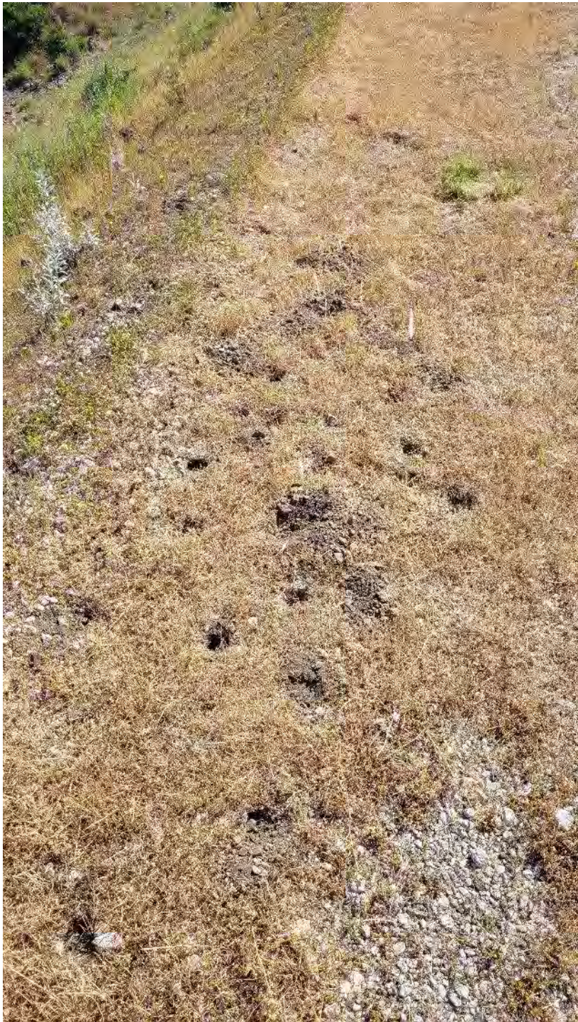
Photo 1: View of rodent holes along the crest of the main dam.
