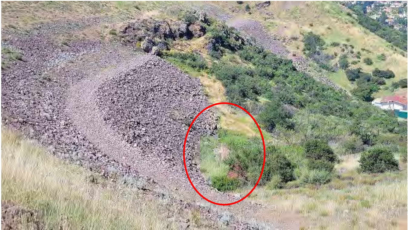
Photo 2: View of the downstream toe of the right side of the main dam. The vegetation was cleared as requested.
